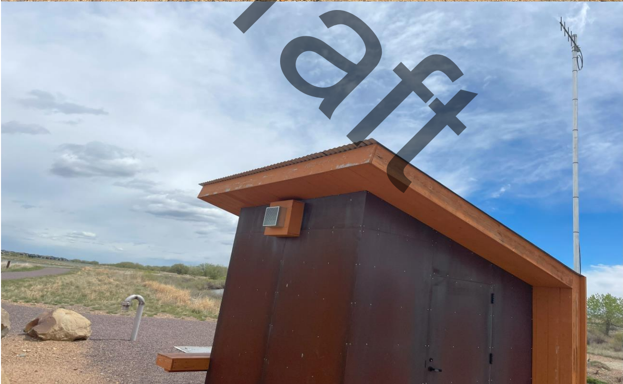
Pump House at the Lakes needs to be repainted. Might be able to have it done this year.
